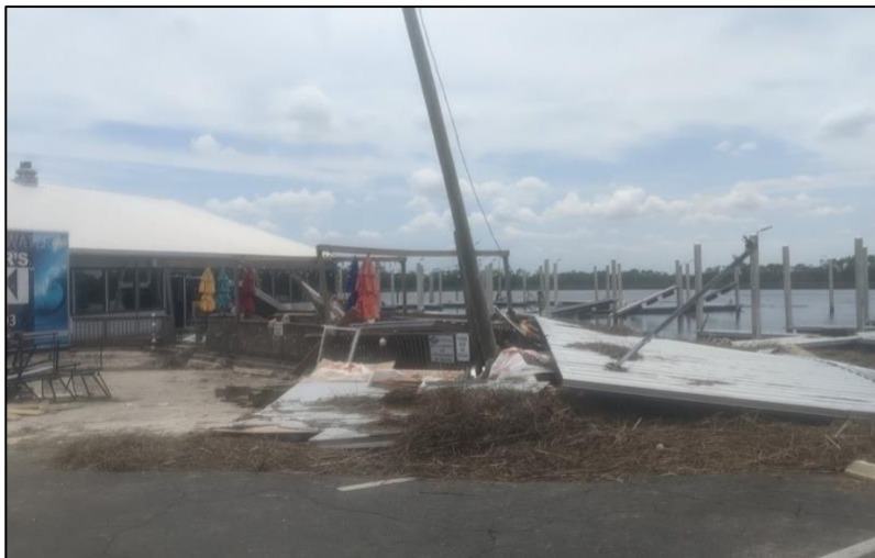
Catastrophic damage to a structure along the Steinhatchee River in Steinatchee, Florida.
